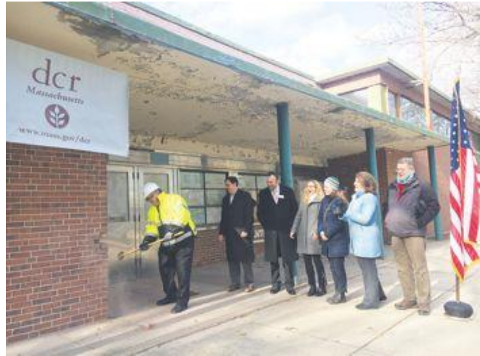
DCR Commissioner with State Rep, EA, CRC, Hill House, and CBI on Demo Day
