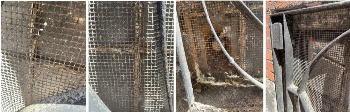
Above (left) - Existing conditions of basement window muntins at 83 Myrtle Street. (Photographs taken Sunday, June 12, 2022).
