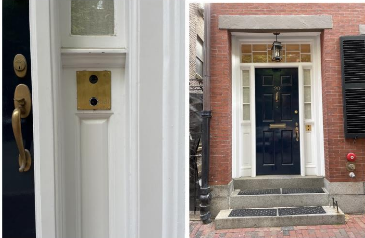
Above - Ring video doorbell (or similar product) approved in November 2020 under conditions that a bronze or brass plate conceal the device except for small holes for the camera and button. Button should not be illuminated though. (Photographs taken on Saturday, June 11, 2022)
