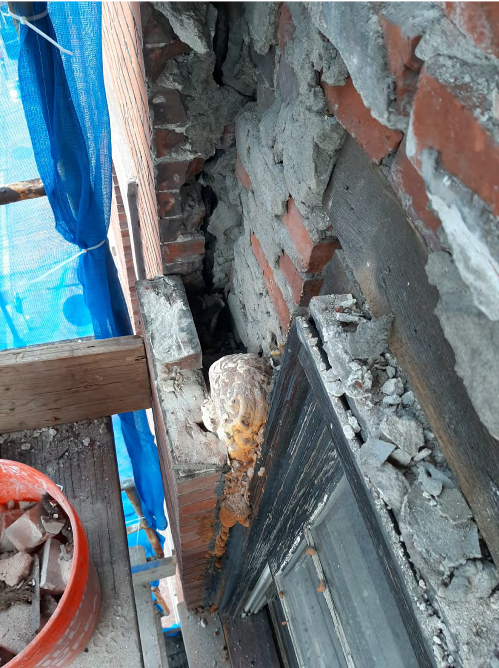
BOWING BRICK FACADE AT WINDOW
