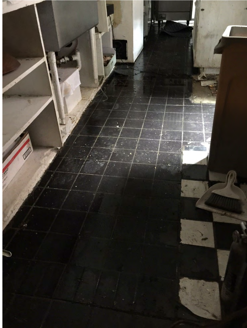
FLOODED KITCHEN FLOOR
