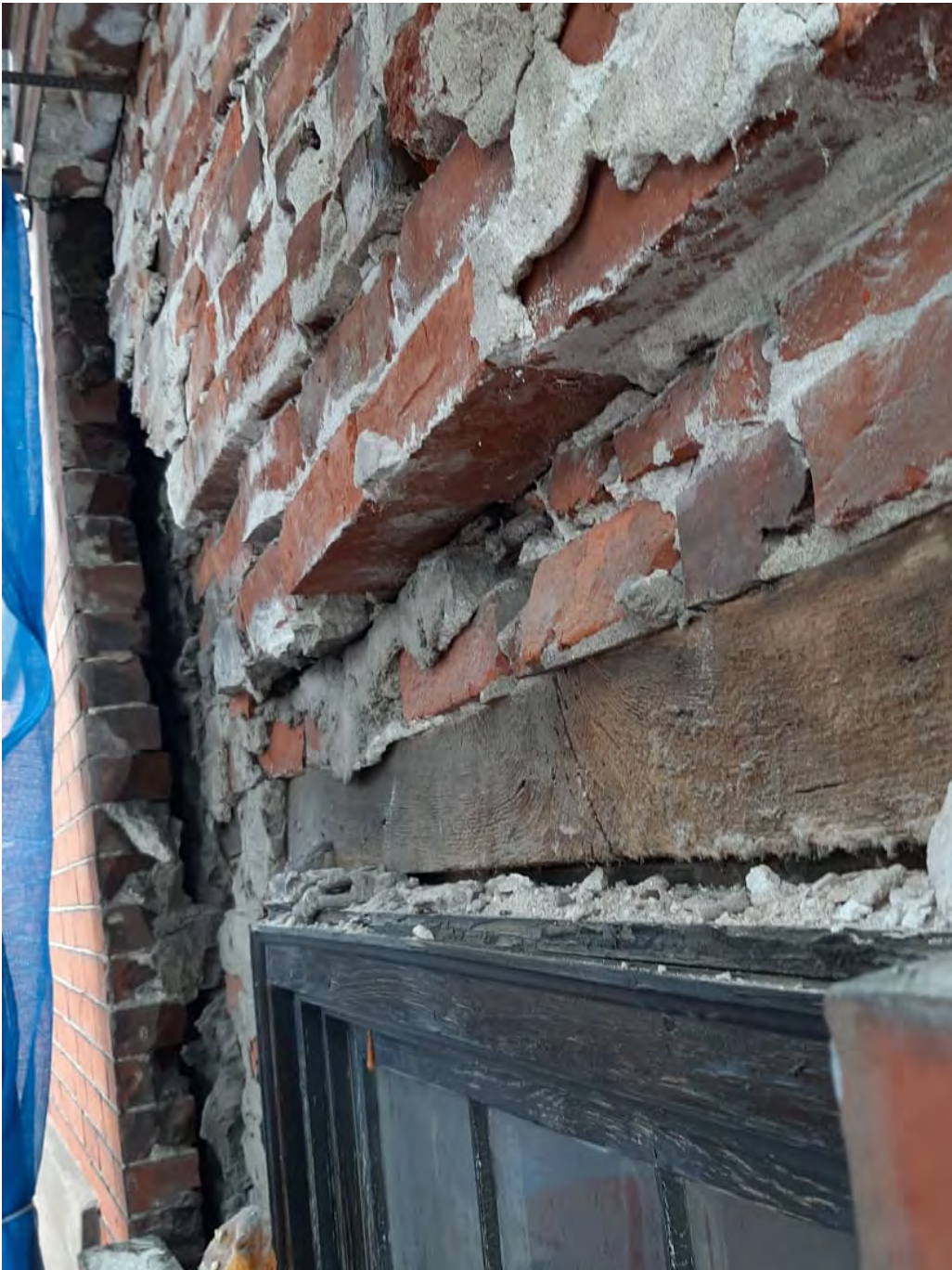
BOWING BRICK FACADE AT WINDOW
