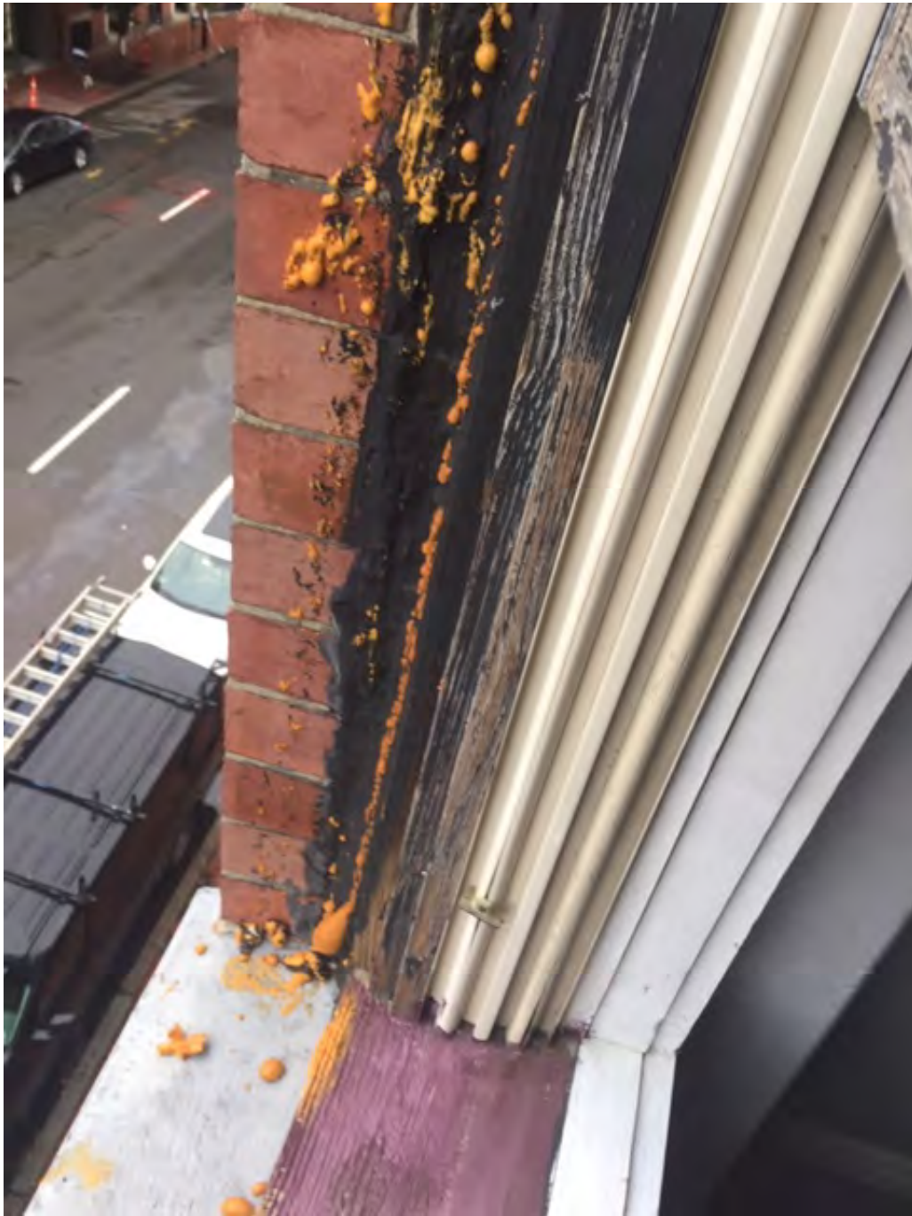
BOWING BRICK FACADE AT WINDOW
