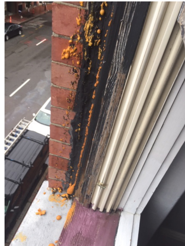
BOWING BRICK FACADE AT WINDOW
