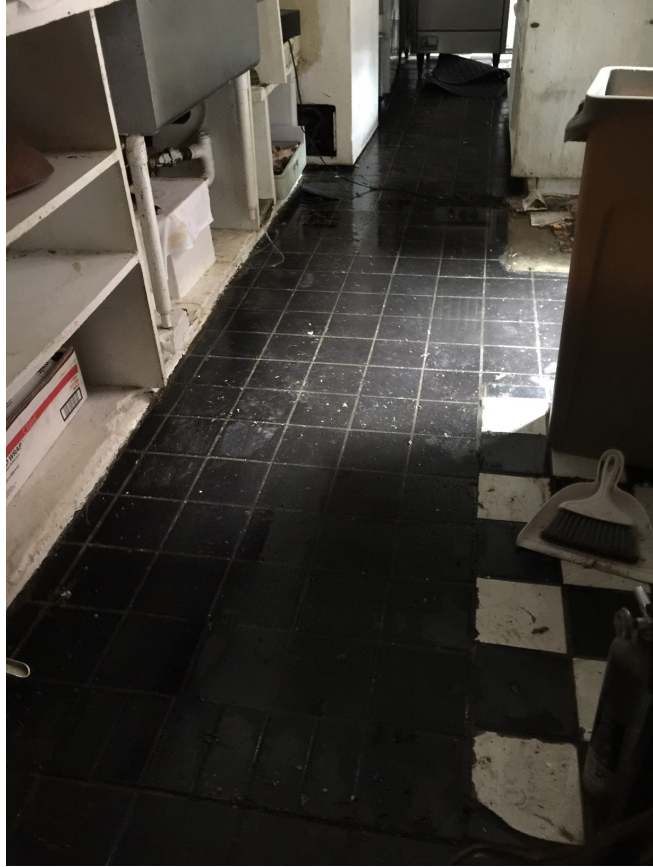
FLOODED KITCHEN FLOOR
