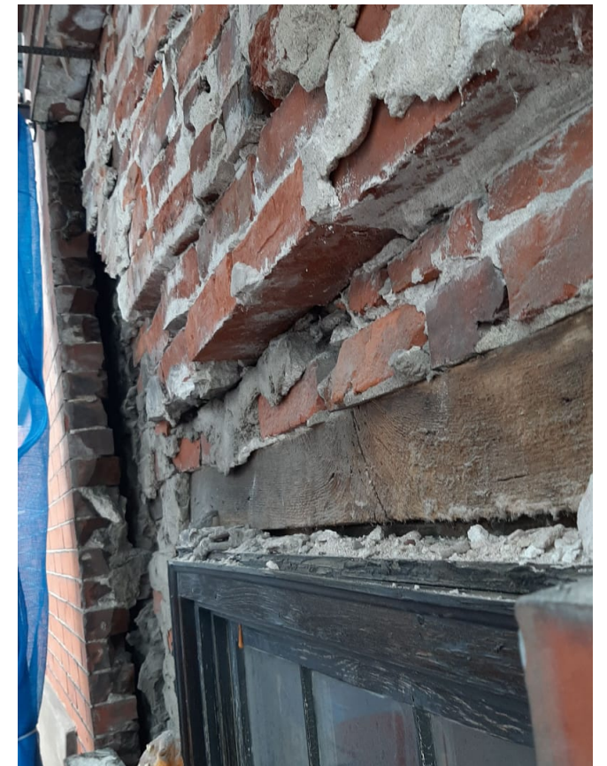
BOWING BRICK FACADE AT WINDOW
