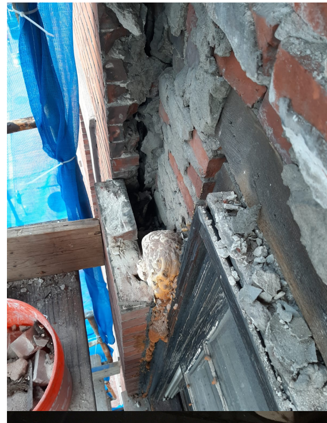
BOWING BRICK FACADE AT WINDOW
