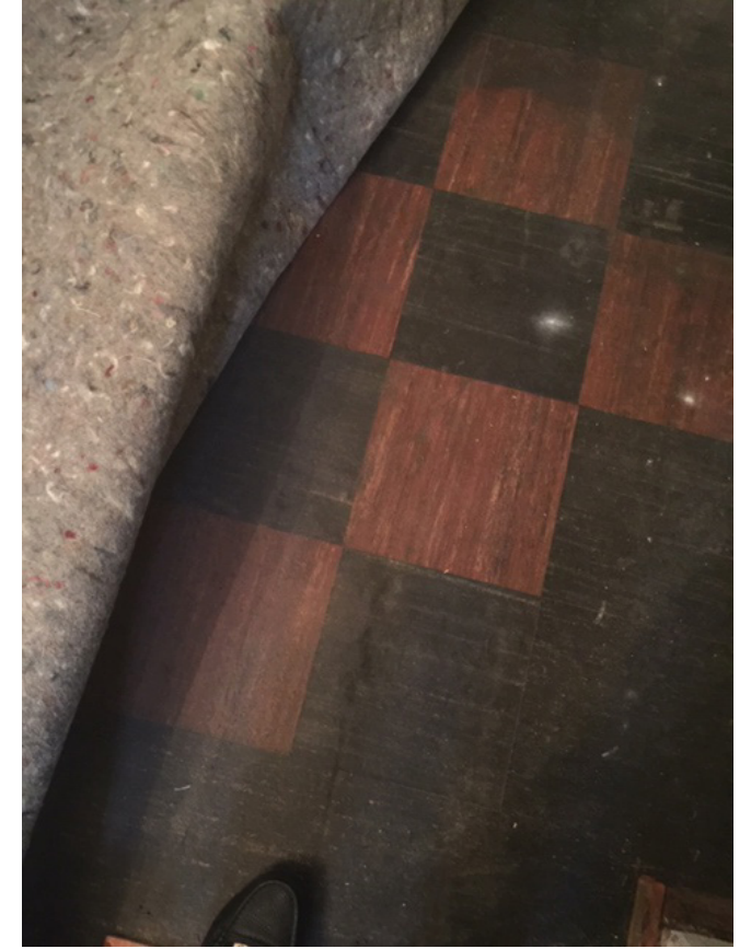
ASBESTOS FLOOR TILE
