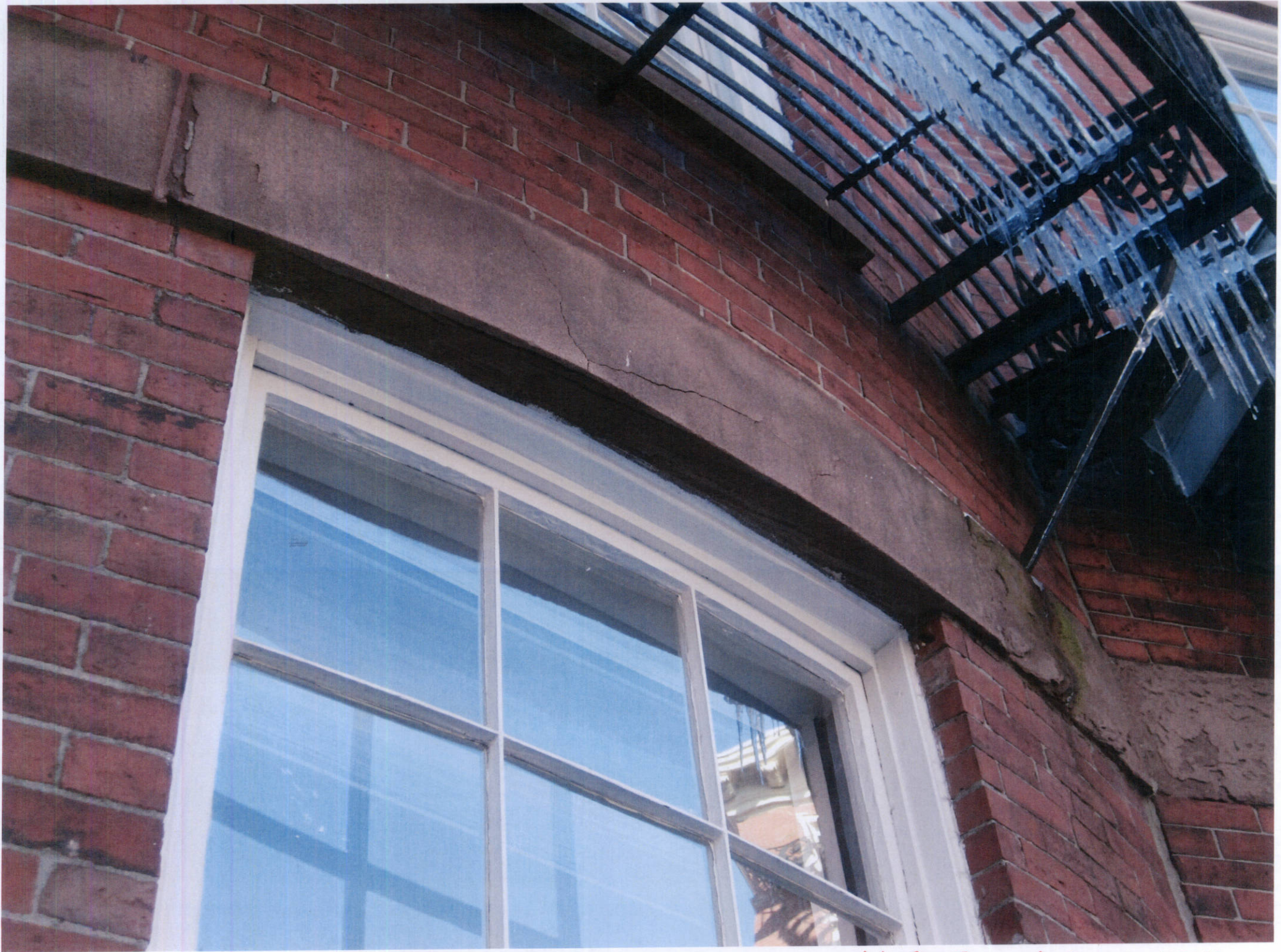
*4 FRONT - DAMAGED BROWNSTONE
