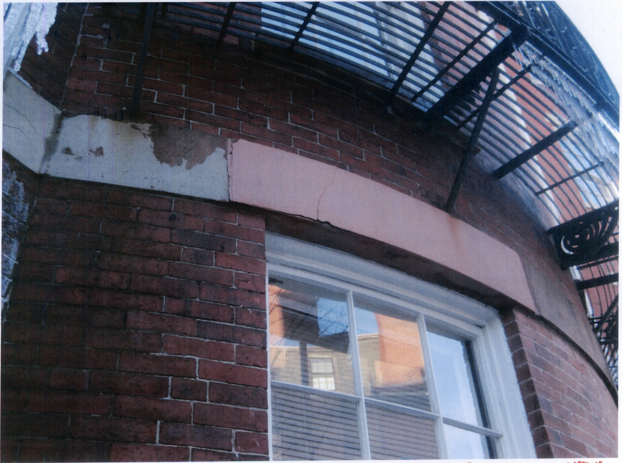
#4 FRONT - DAMAGED BROWNSTONE
